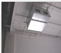
Toll Process Space Cooling & Heating Air Handling Units
