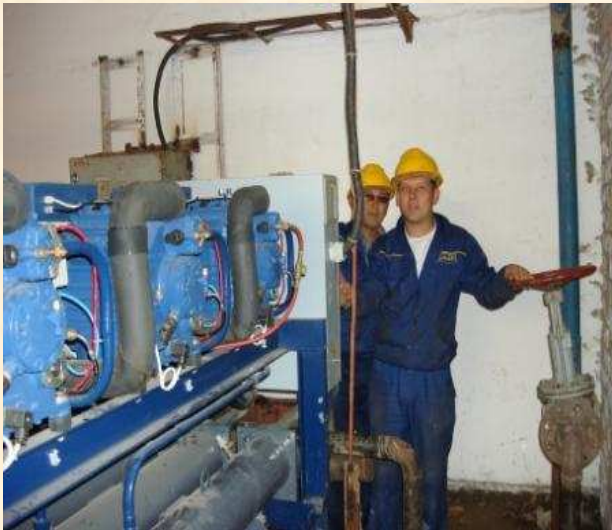
Chiller in hydrogen recovery factory Power 32 KW R404a 2009
