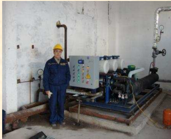
Chiller in air separation factory Power 47 KW R404a 2009
