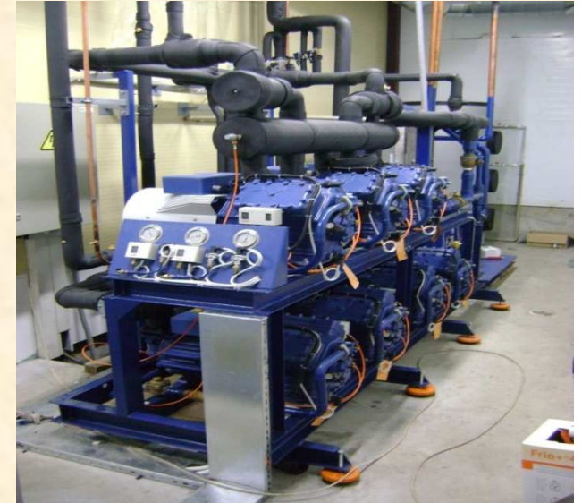
Refrigerating plant at supermarket Medium temperature Power 224 KW R404a Low temperature Power 48 KW R404a
