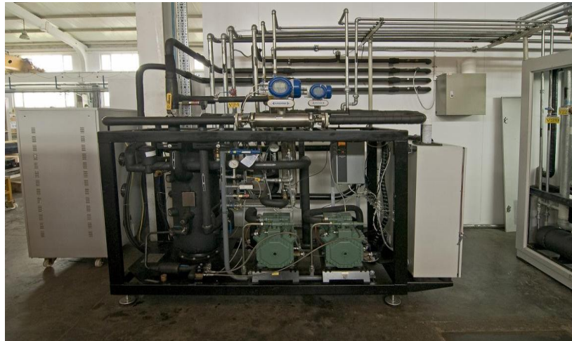
Figure 24. CO 2 refrigerant preparation unit [27]
