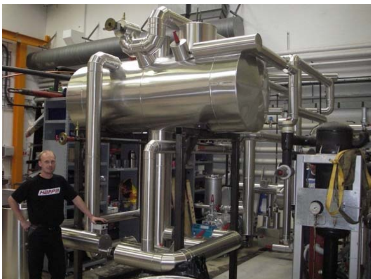
100 kW industrial low temperature CO 2 plant used for testing and training
