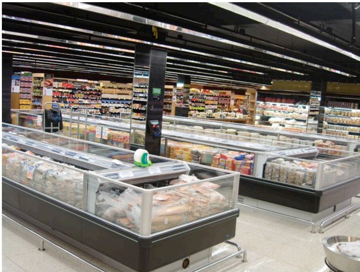
The frozen products section of the new store: Low temperature islands with CO 2
