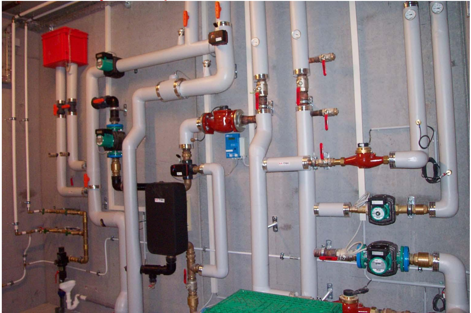
Heat recovery installation
