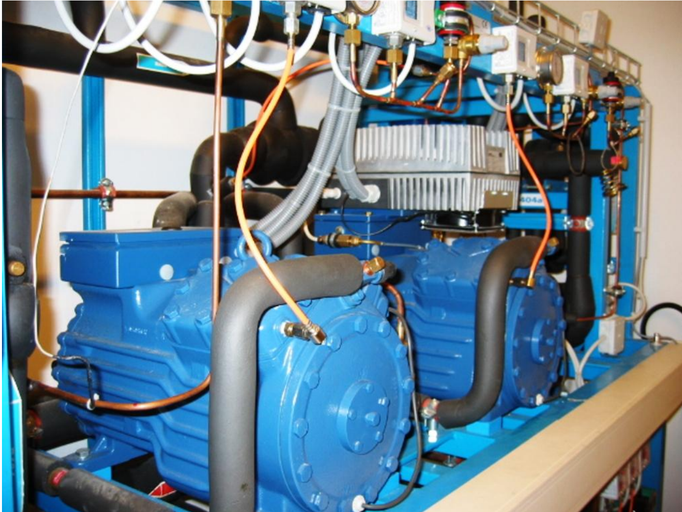
Bock compressors showing variable speed controls
