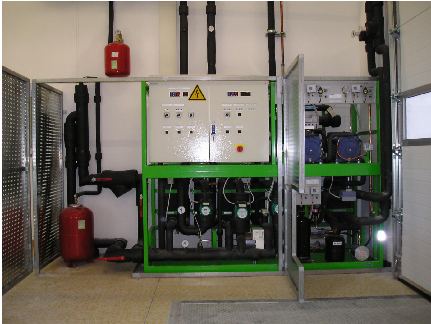
Control unit with heat pump, process cooling and heat recovery
