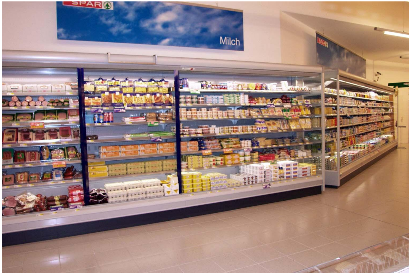
Refrigerated display units in SPAR store
