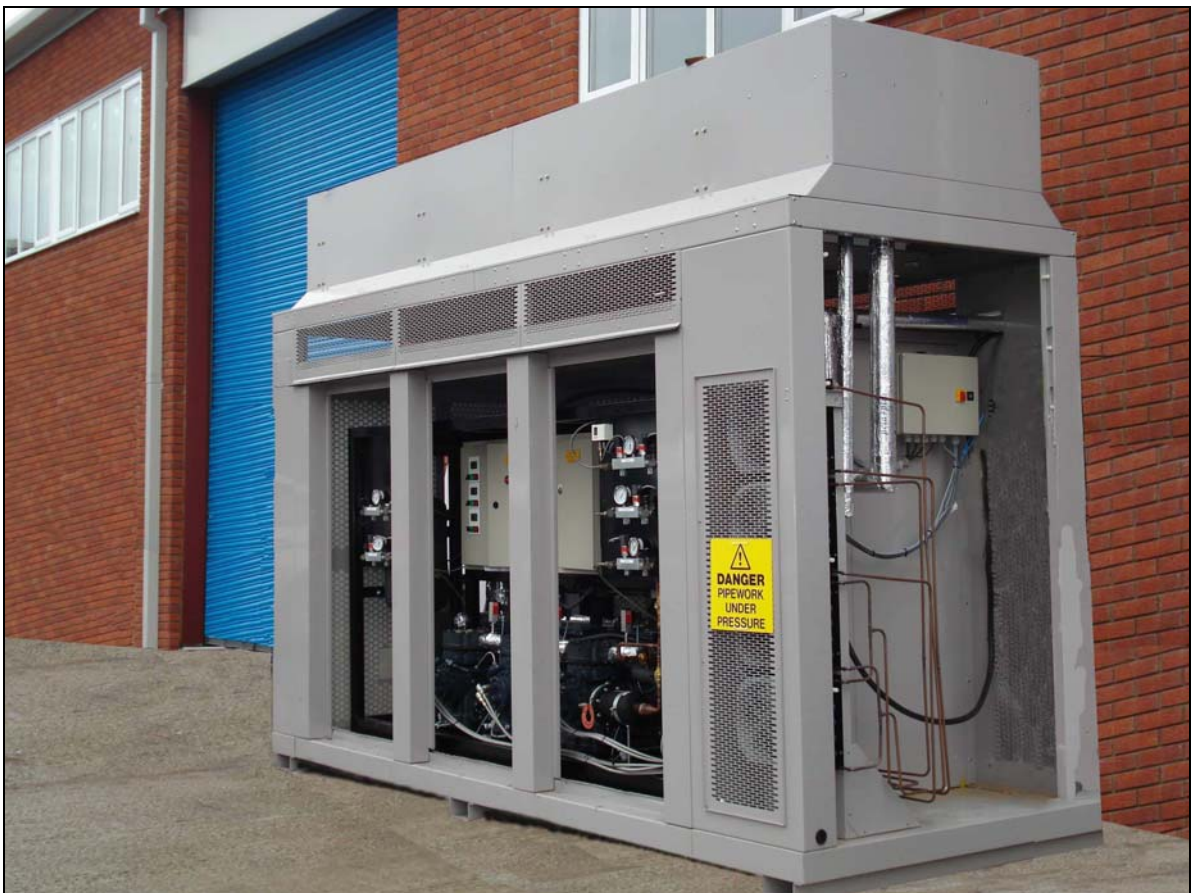
Figure 7. Space Engineering Services Trial Plant
