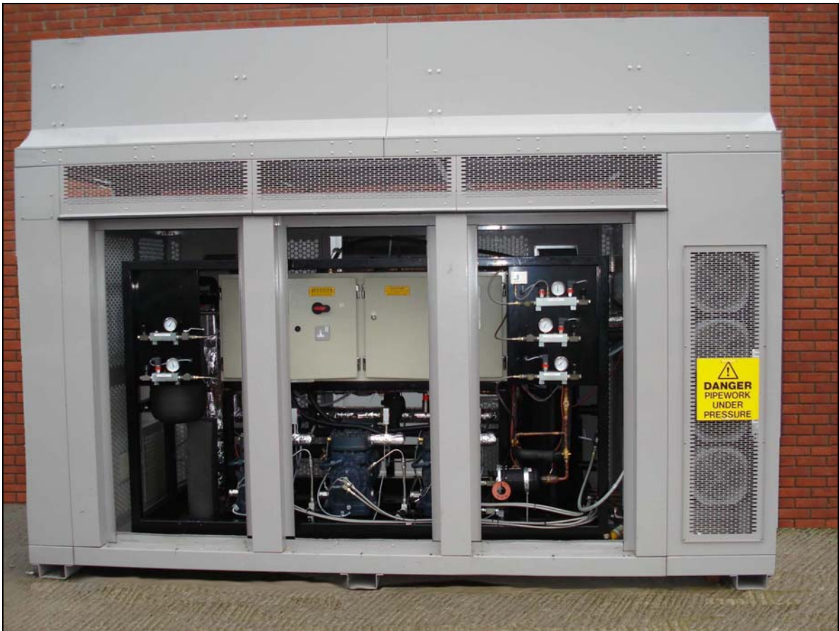
Figure 6. Space Engineering Services Trial Plant
