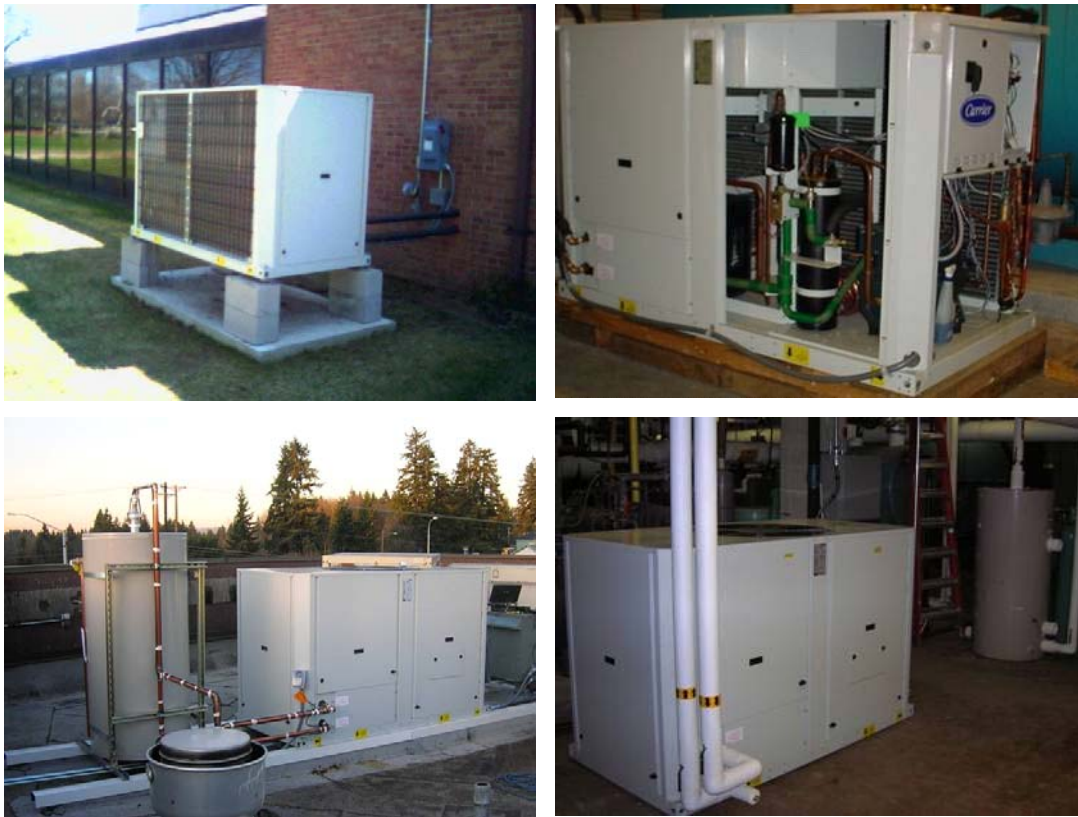
Figure 2: Installed CO 2 Heat Pump Water Heaters
