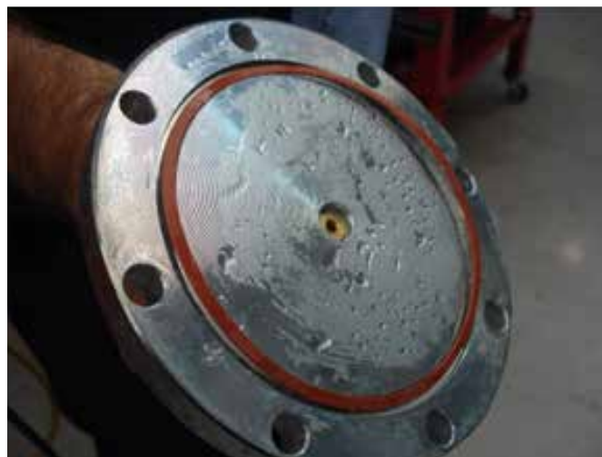
Figure 30. Example of moisture on the flange of a drier
