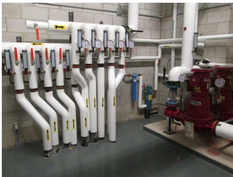
Figure 19 A geothermal well in the ice rink North Wentworth Arena, Hamilton, ON.
