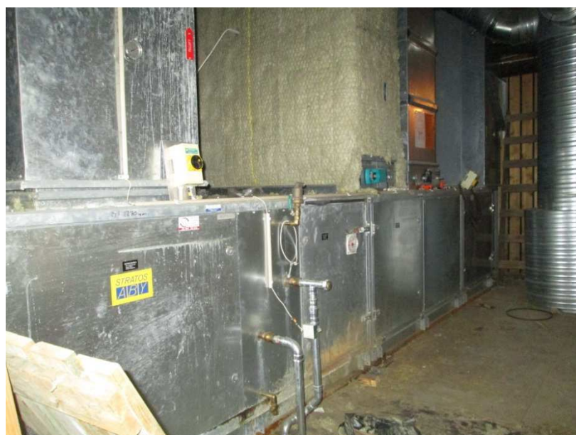
Figure 29 The original ventilation unit in the ice rink from 1985.
