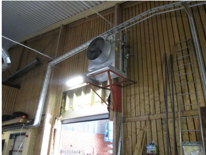
Figure 30 The original fan-coils in the ice rink from 1985.
