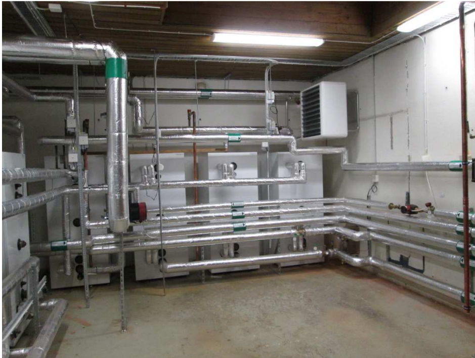
Figure 27 A view of the technical room containing the heat recovery system.
