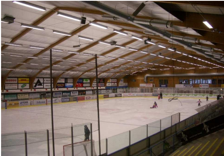
Figure 6 Example of an ice rink with a light tube installation.
