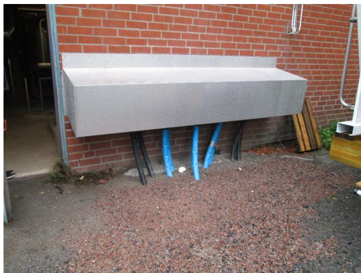
Figure 35 Collection point for the geothermal wells outside the machine room.
