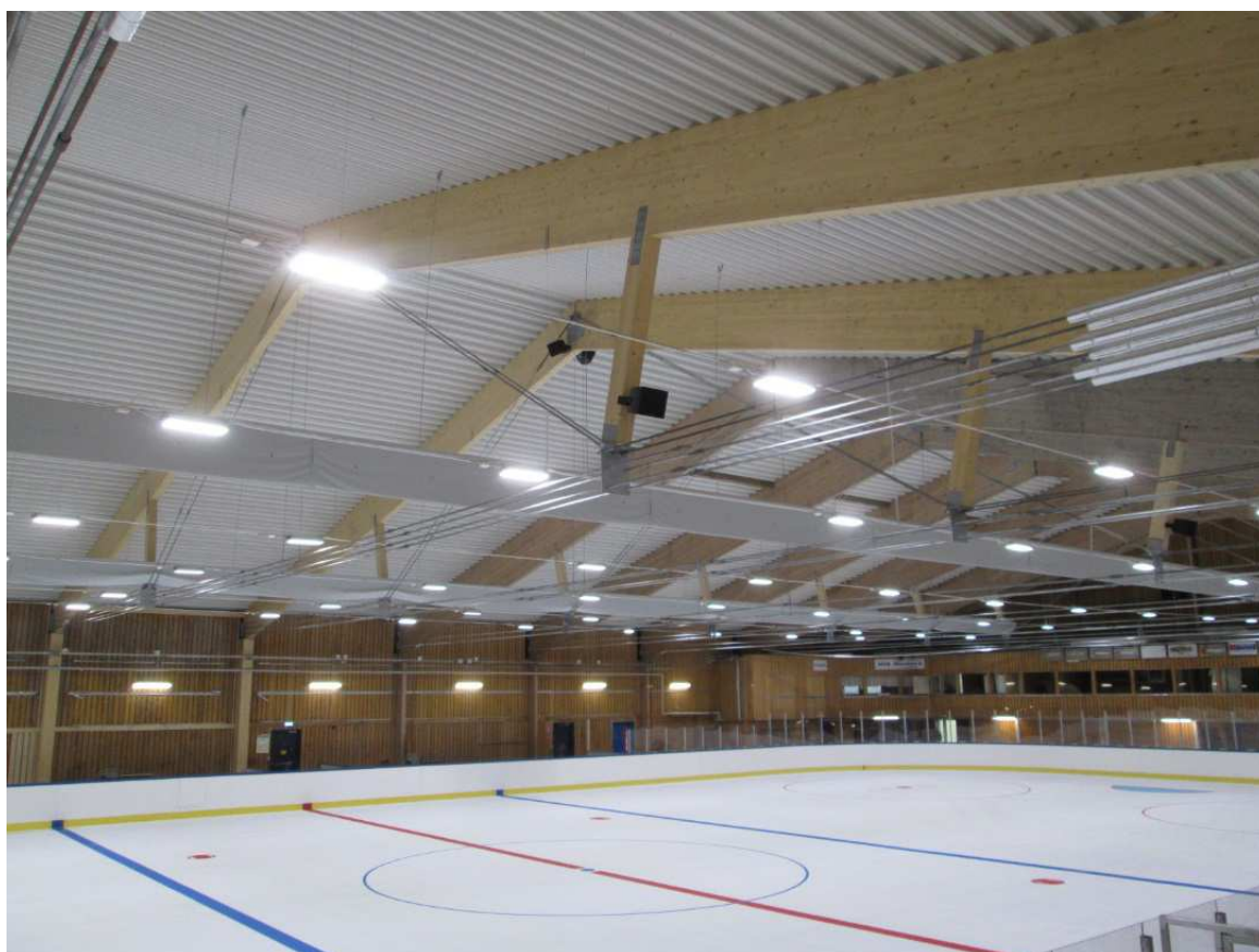
Figure 33 LED lighting system of Gimo ice hall.
