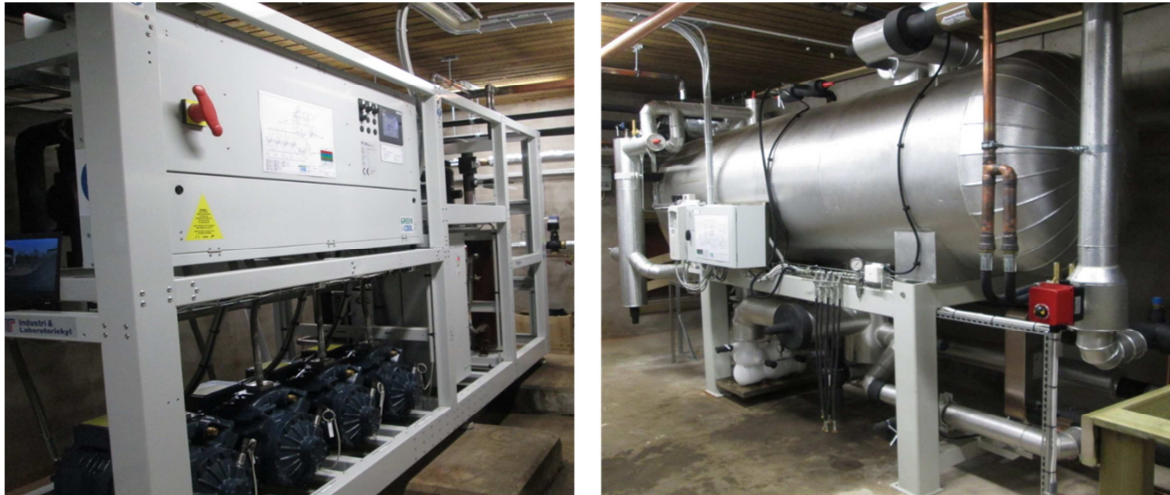
Figure 25 Overview of the refrigeration system in the GIMO ice rink.
