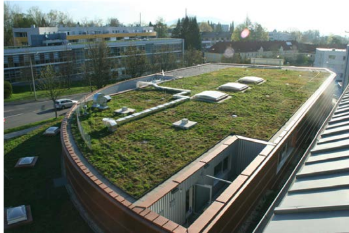
Figure 6 Green roof on a supermarket in the residential area of Linz (Austria) (Built to Bloom, 2015)
