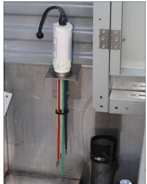
Electric Water Level Control
