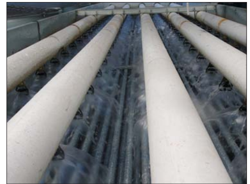
Spray Water Distribution System
