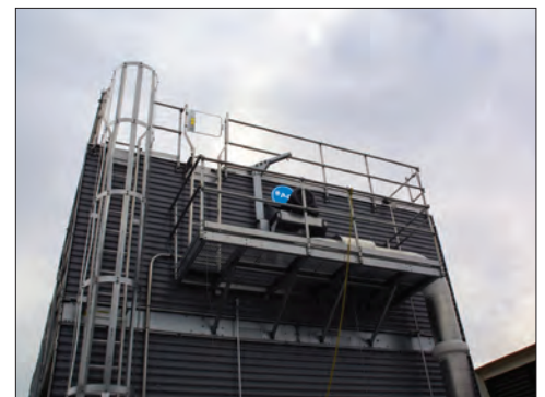
External Motor Platform, Ladder, Handrails, and Safety Cage
