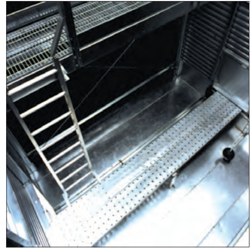
Internal Ladder, Service Platform, and Walkway
