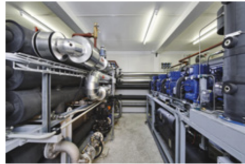
Heat pumps with GEA Bock CO 2 compressors
