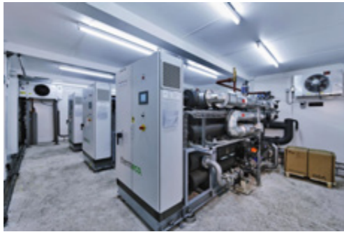
Heat pump in the abattoir of Zurich
